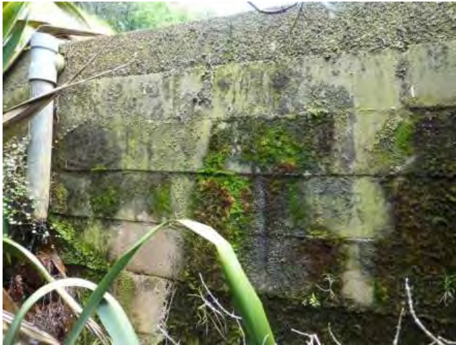
Figure 60: Mosses growing on the face of the Lower Emergency Dam
