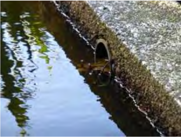
Figure 15: Outlet pipe from Lower Emergency Dam
