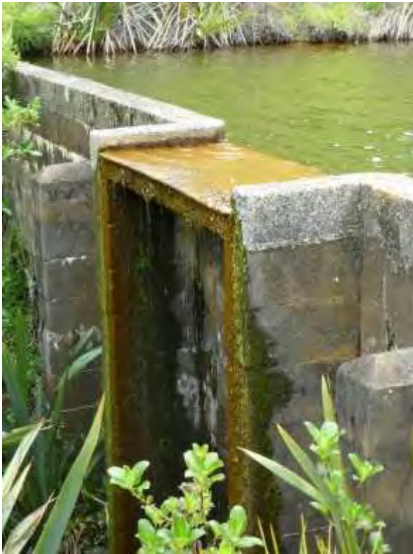
Figure 9: Spillway structure on Upper Emergency Landing Dam, showing 'perched' overhang
