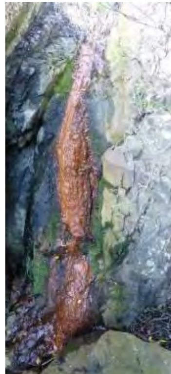
Figure 53: Damp flow down the rock face at the bottom of the catchment
